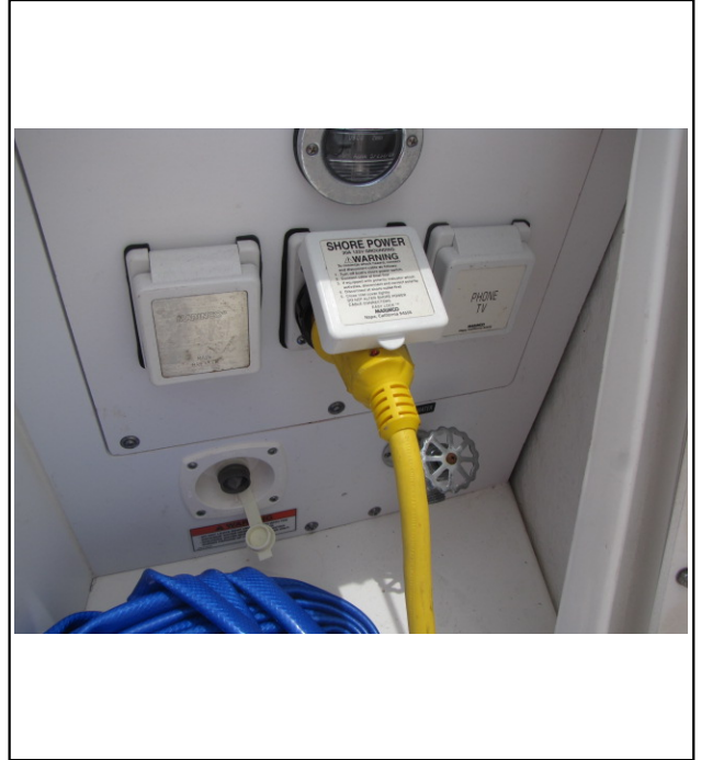
Shore power connection & breaker, photo 43.
