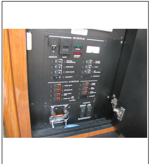
Electrical panel, photo 12.
