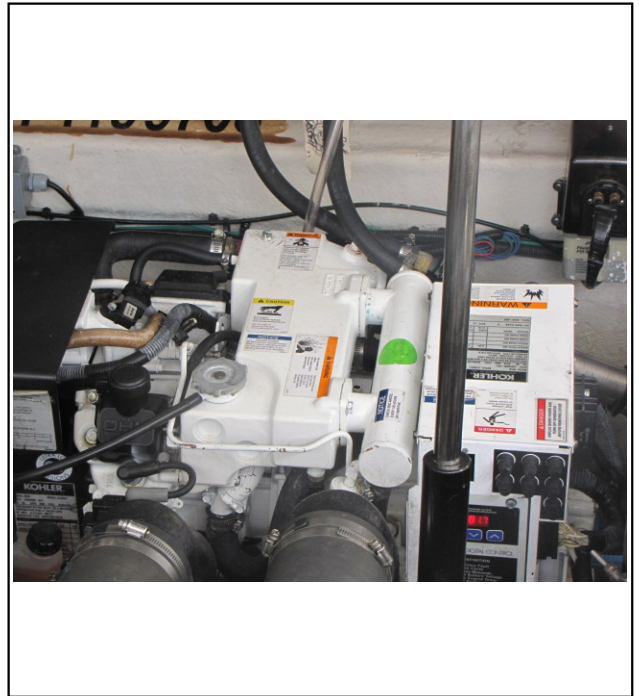
Kohler generator, photo 28.
