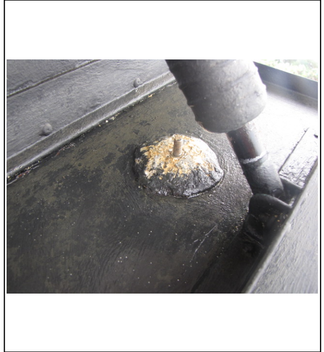
Starboard Trim tab zinc, photo 22.
